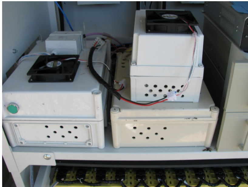
Figure 10. BESS Communication Module.
