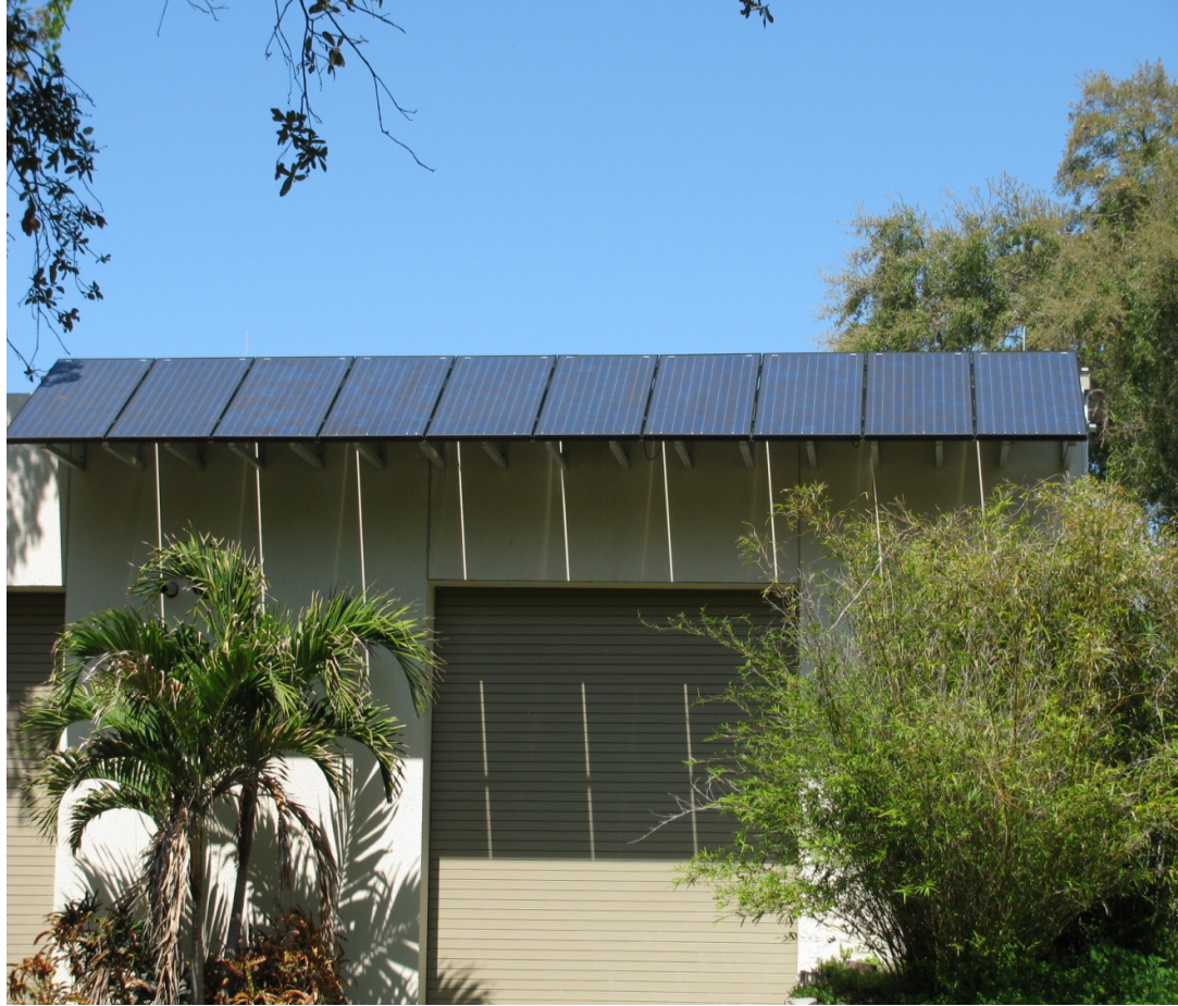
Figure 20. Solar Installation at USF St. Petersburg
