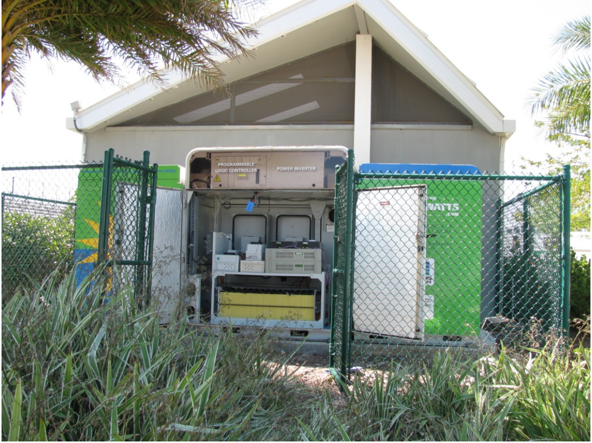
Figure 14. LiFePO4 Unit Enclosure
