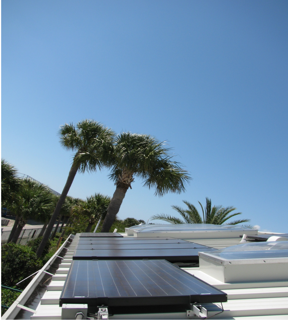
Figure 19. Solar Installation at Albert Whitted Park
