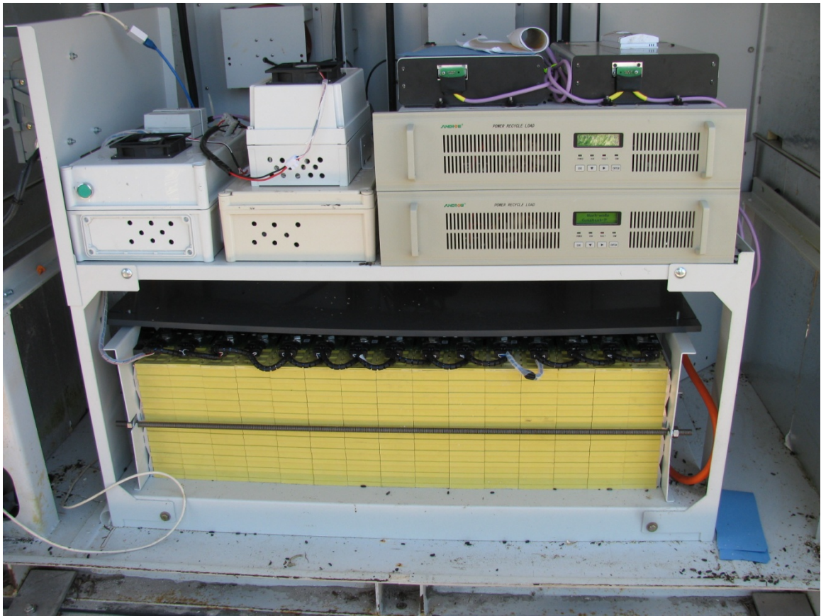
Figure 21. LiFePO4 Unit with BMS
